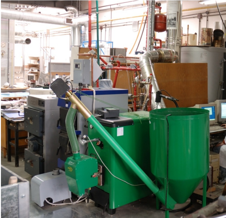
Fig. 3. View of the heat station located in a laboratory belonging to the Poznan University of Technology (Division of Heating, Air Conditioning and Air Protection, Institute of Environmental Engineering)
