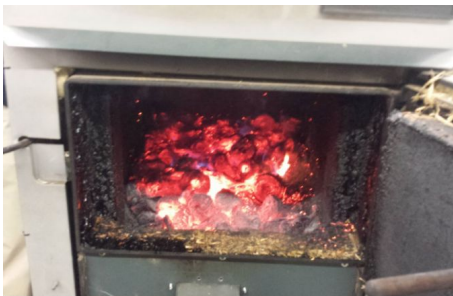
Fig. 3. View of the gasification chamber with open loading door
