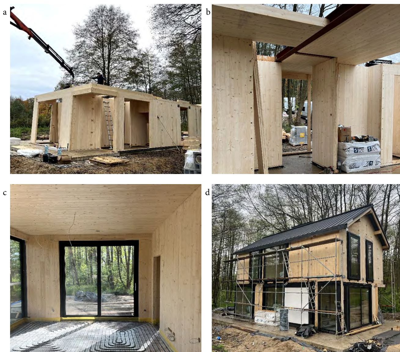
Fig. 1. The construction site of a wooden detached house using the CLT system in Oświno (PL): (a) assembly of CLT panels, (b) interior finishing of CLT panels, (c) floor heating installations in the wooden interior, (d) construction of the house in its raw state. Photo by Natalia Paszkowska-Kaczmarek
